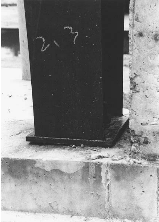
FIGURE 16.10 A gap under the column base plate.
